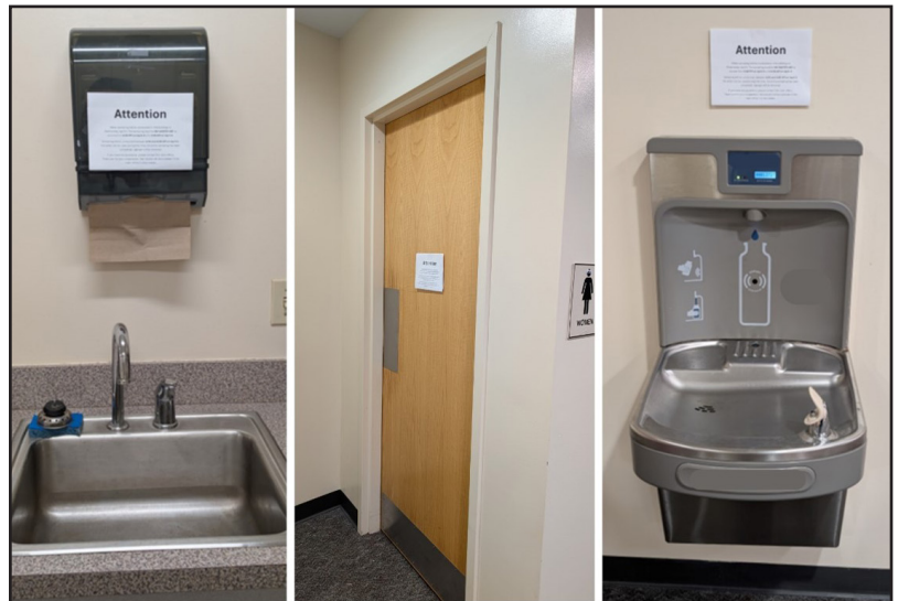
Figure 4. An example of signs posted throughout a building alerting building users of upcoming sampling. Signs are posted above each point of potential water usage including handwashing sinks, bathrooms, and filtered bottle-filling stations.
